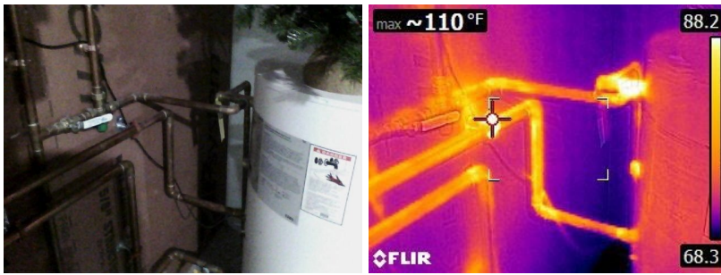
IR Hot Water Heater Operation
