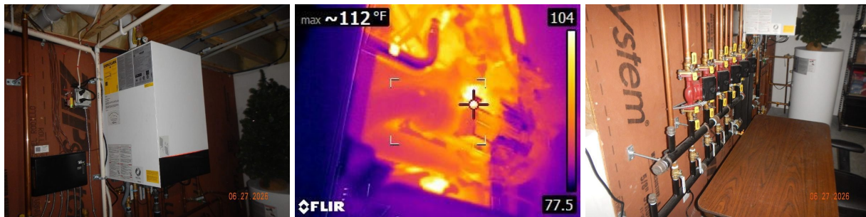
Interior Boiler Heat Tracing
