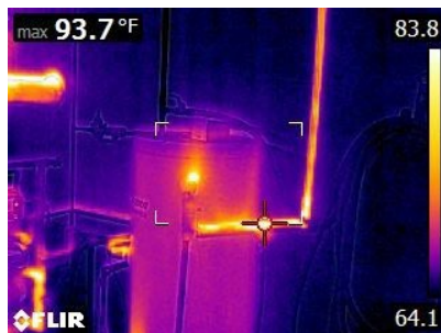
IR Hot Water Heater Heat Tracing
