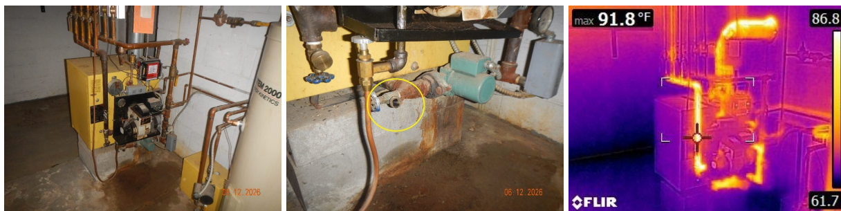
IR Boiler Operation
