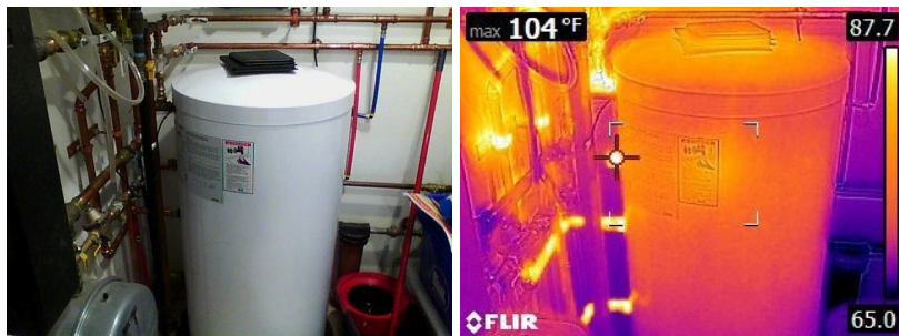
IR Hot Water Heater Operation
